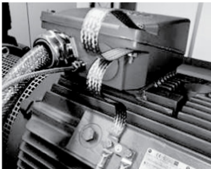
Illustration 10: Installation of EMC straps from the Terminal Box to the Motor Frame
