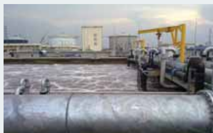
Wastewater treatment, Hanoi, Vietnam The wastewater treatment plant, Yen So Park, treats 50% of Hanoi's wastewater. More than 90 VSDs are installed, of which 12 450 kW VLT® AQUA Drives control the blowers.
